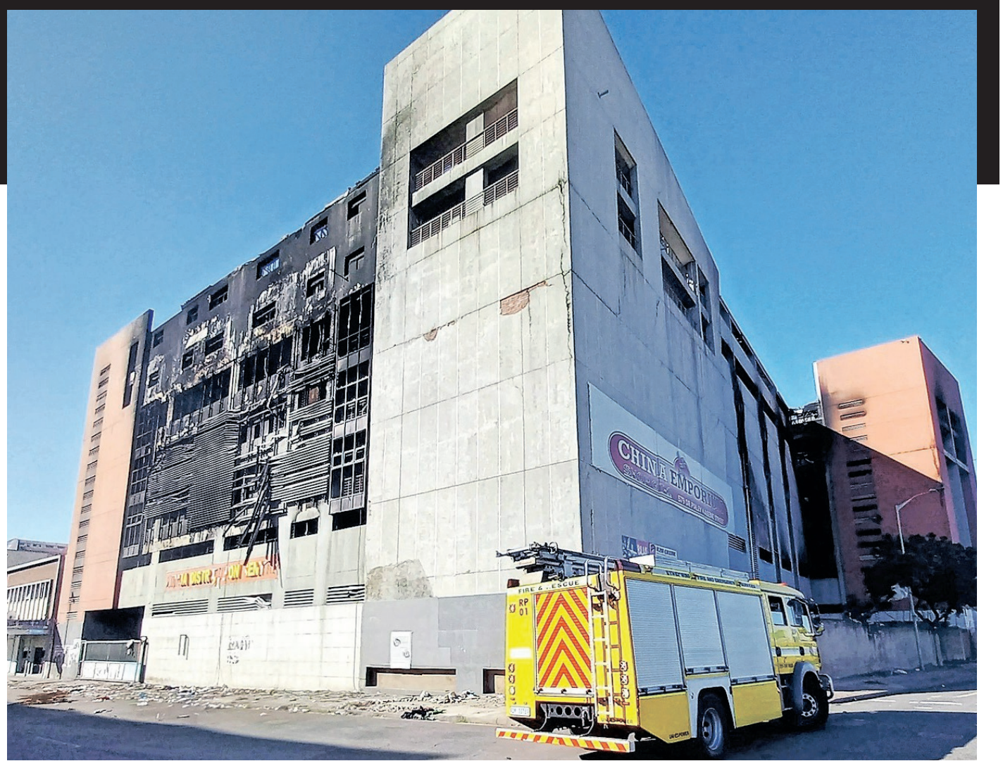
THE China Emporium building in the Durban CBD, seen in a picture last year, is set to be demolished after it was severely damaged in a fire in January last year. | TUMI PAKKIES African News Agency (ANA)
